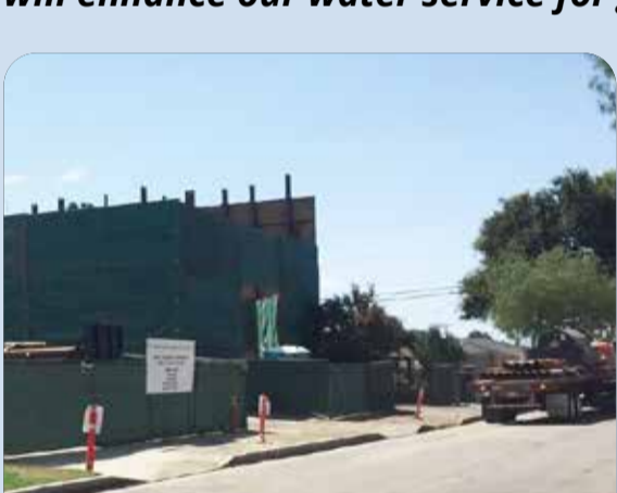
The Leahy Well, a new water supply source for Bellflower, located at 14742 Leahy Avenue
